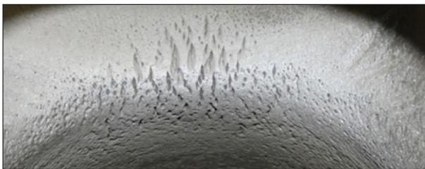
Figure 1. Cavitation occurs when rapid changes of pressure in a liquid lead to the formation of small vapour-filled cavities (air bubbles) and can ultimately lead to cracking or module washout.
